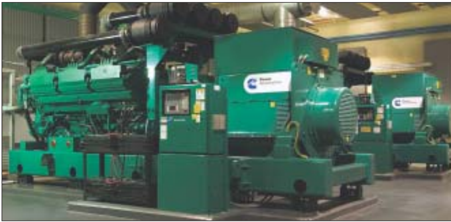
Two PowerCommand 2.7-megawatt diesel generator sets provide back-up power for a water treatment plant in Wyoming, Michigan.
